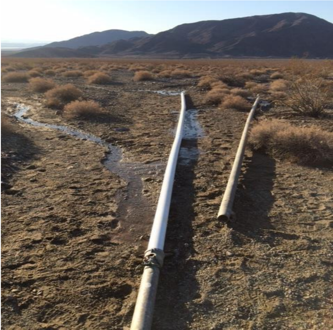
Figure 5. Discharge pipe for well project at Soda Mountain Solar Project.
