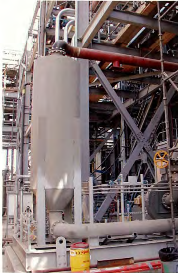
Figure 1-2 Vaporizer at the Elk Hills Power Plant
