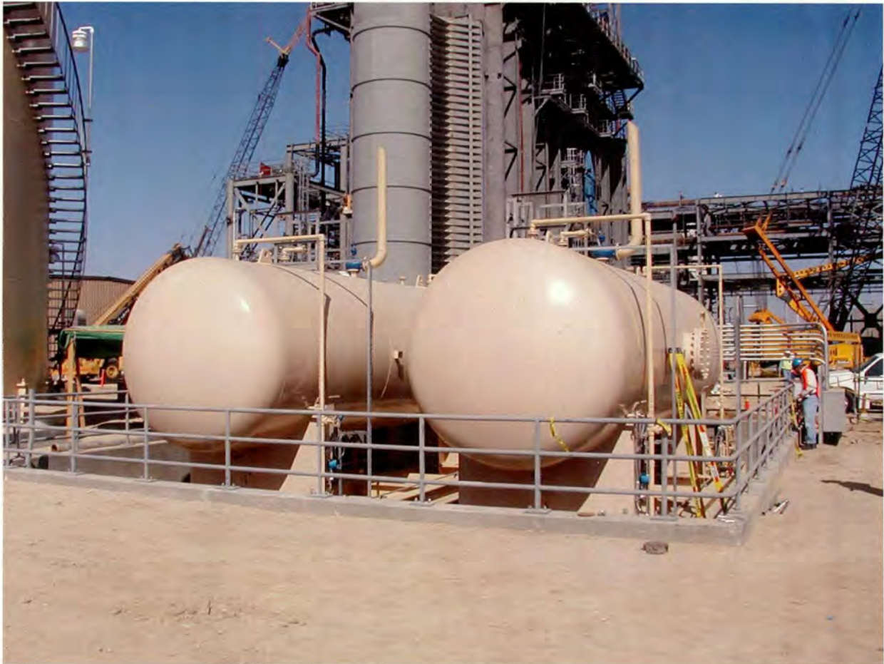
Figure 1-1 Aqueous Ammonia Storage Tank and Containment Structure
