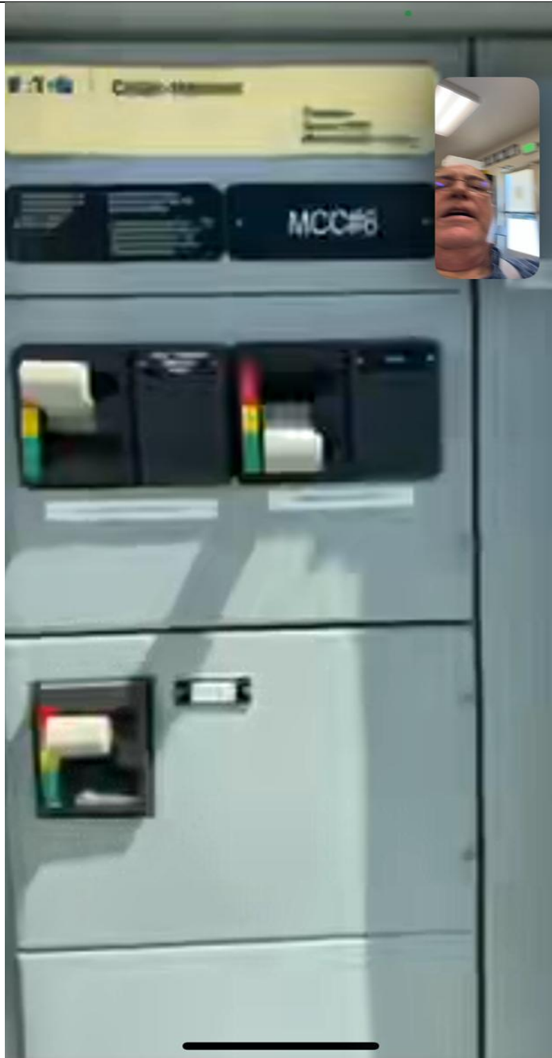
Photograph #1: Labeled MCC#6
