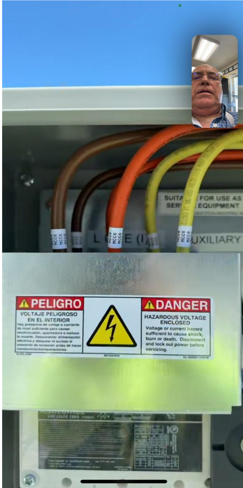
Photograph #4: Labeling of conductors inside Transfer switch
