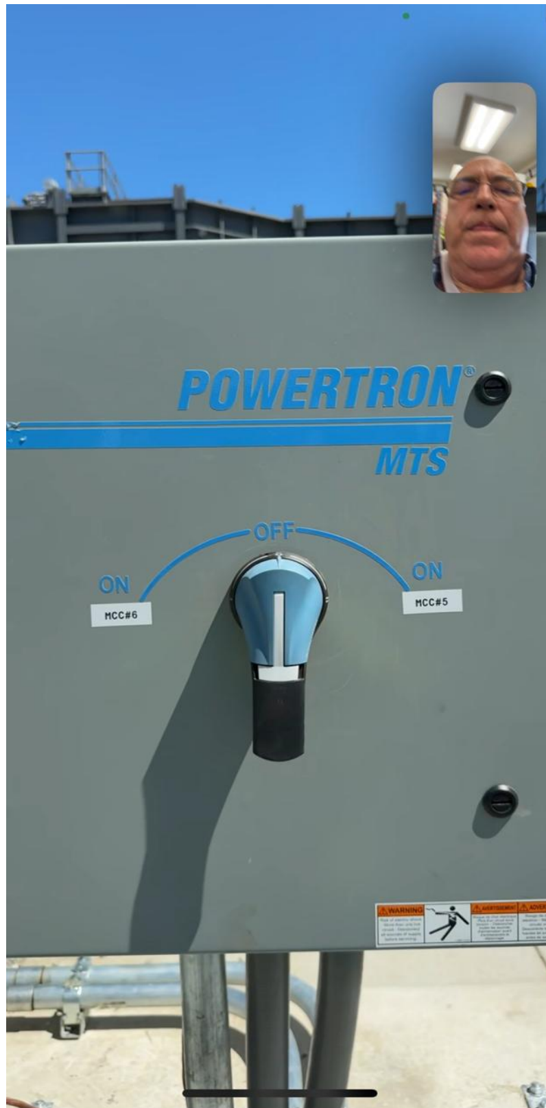
Photograph #6: Labeling of Manual Transfer Switch
