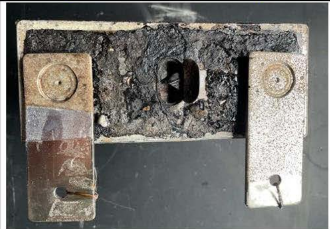
Figure 34: After thermal runaway-3
