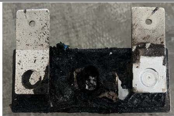
Figure 22: After thermal runaway-3
