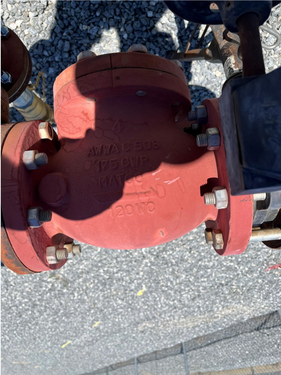
Photograph #8: Check valve.
