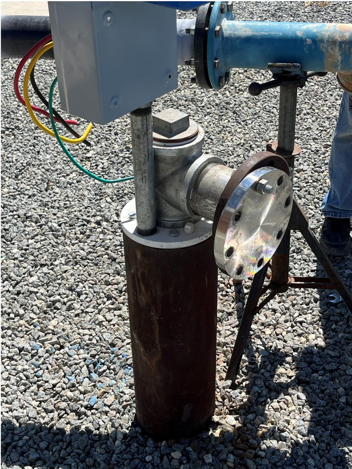
Photograph #6: New Well Head.
