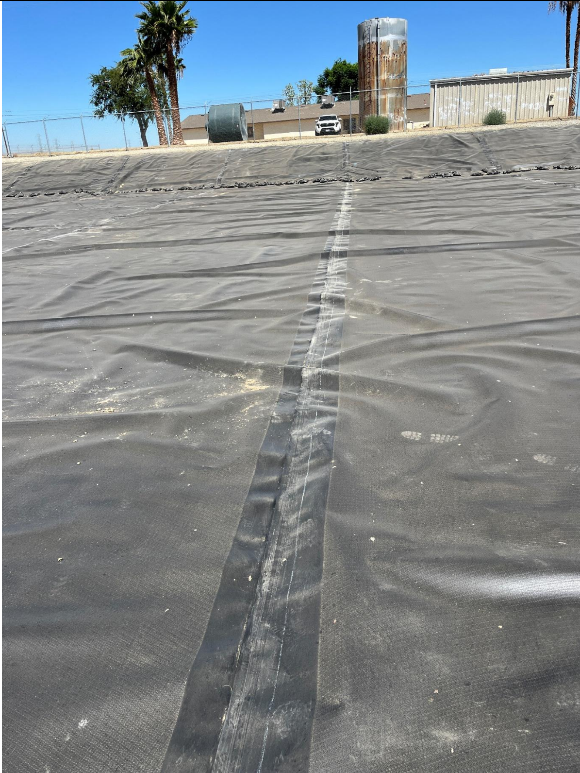
Photograph #11: Typical double weld seam. (3 rd party testing pending)
