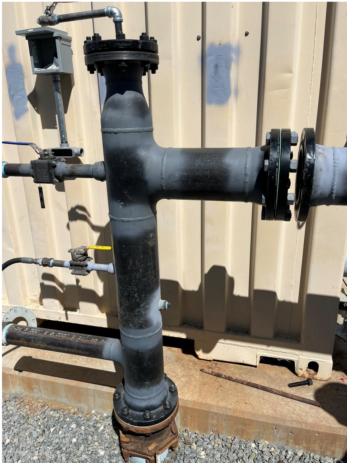
Photograph #3: Demineralizing trailer isolated end of test.
