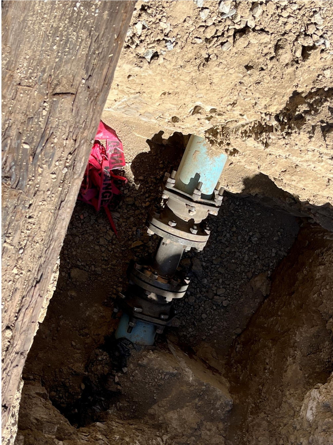
Photograph #5: Existing thrust block and blind plate flange isolating from old well.
