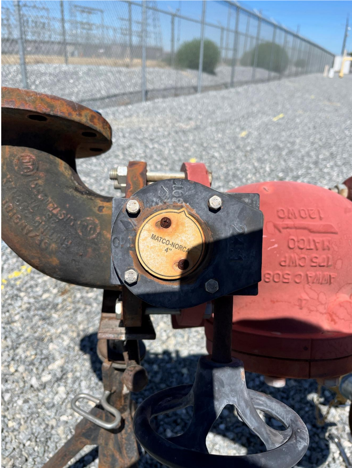
Photograph #9: Gate valve at wellhead assembly.
