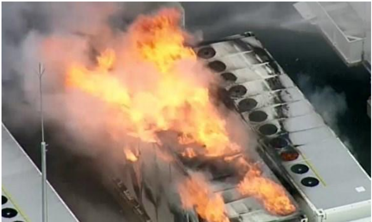
Figure 5. Engulfed Battery container at the Victoria BESS facility in Australia in 2021.
