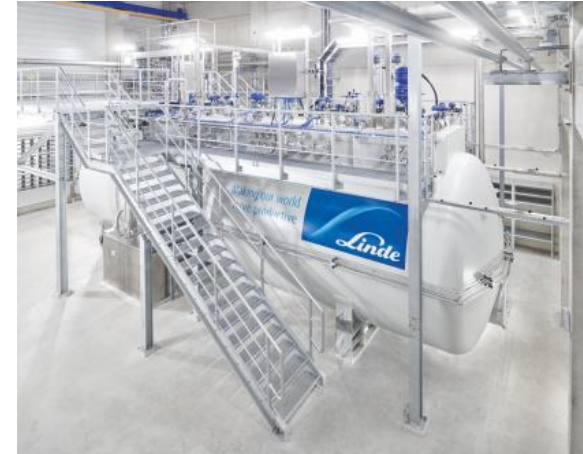
Linde H 2 liquefaction plant
