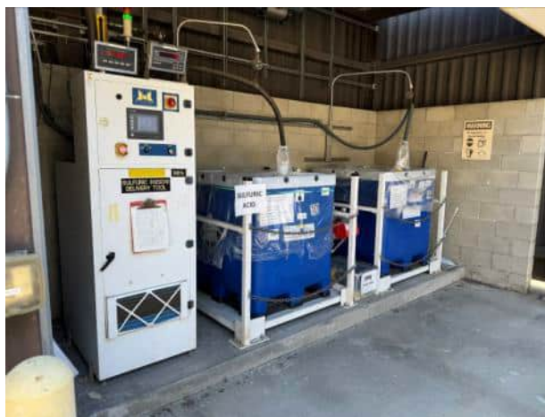
28. View of acid storage
