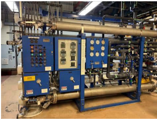
13. View of the water and wastewater treatment systems
