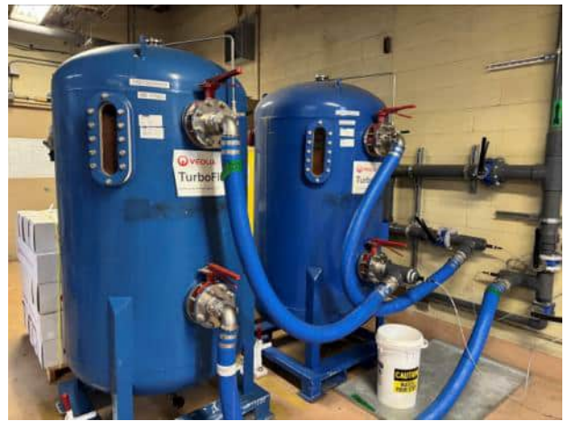
14. View of the water and wastewater treatment systems
