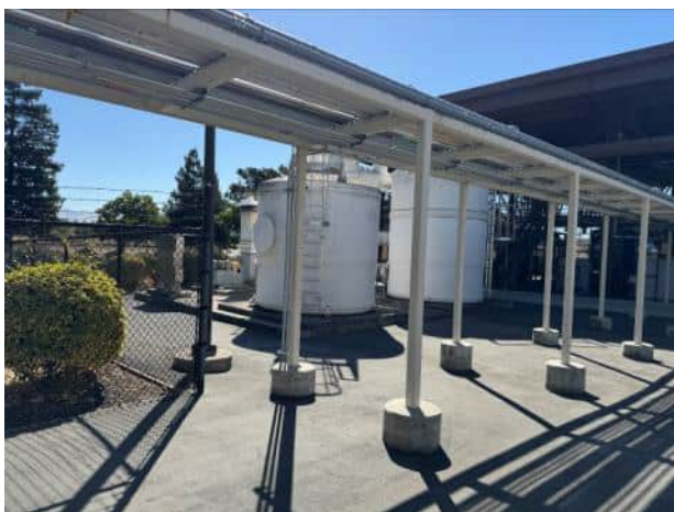
27. View of GAC tanks
