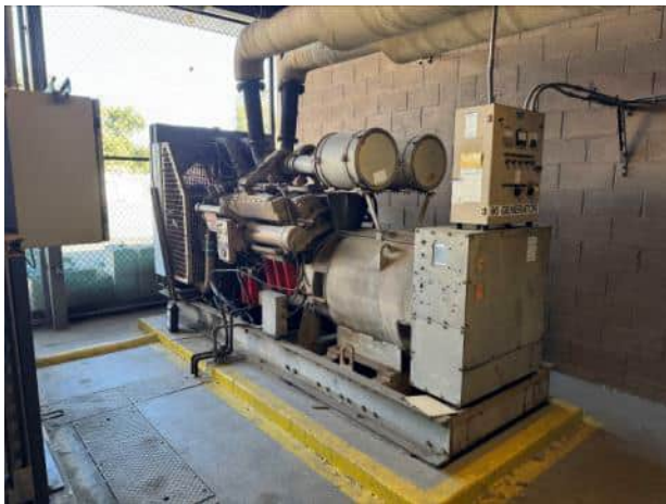
19. View of an electrical backup generator
