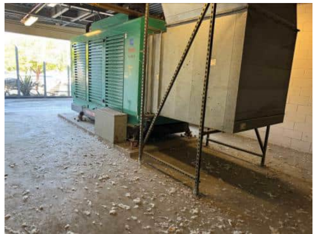
16. View of an electrical backup generator
