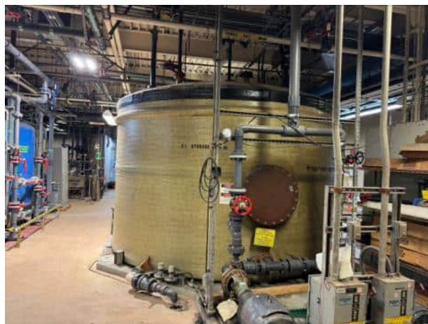
12. View of the water and wastewater treatment systems
