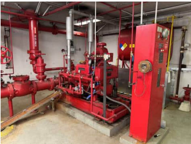
35. View of the fire pump
