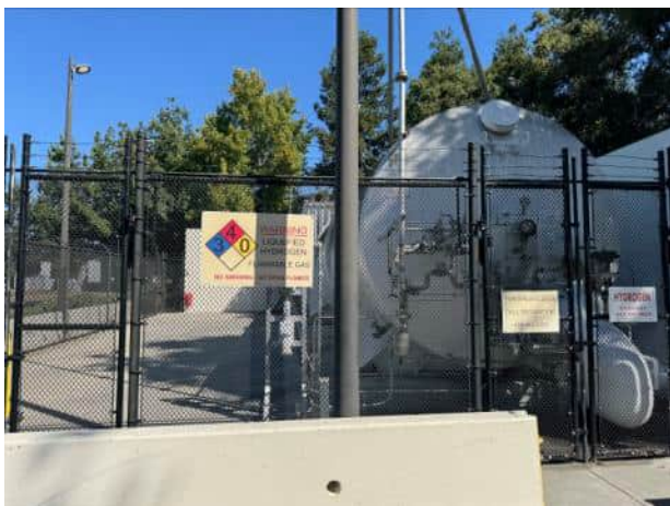
29. View of the liquid hydrogen tank
