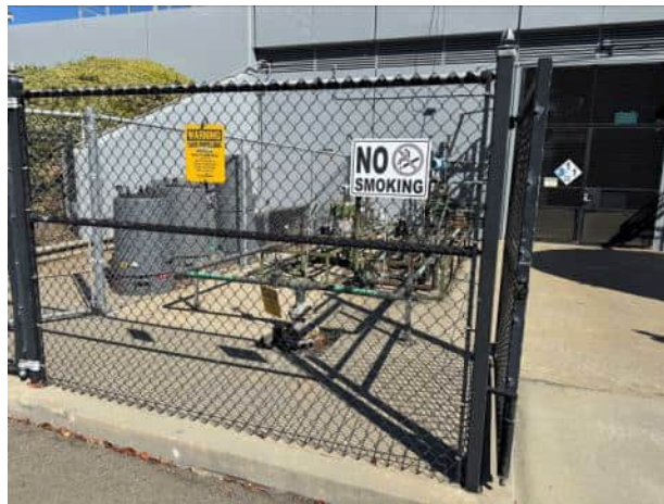
20. View of incoming nitrogen pipeline equipment
