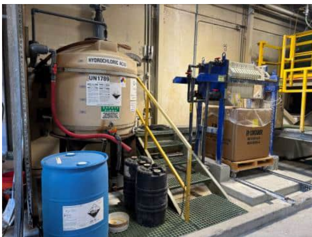
9. View of the water and wastewater treatment systems
