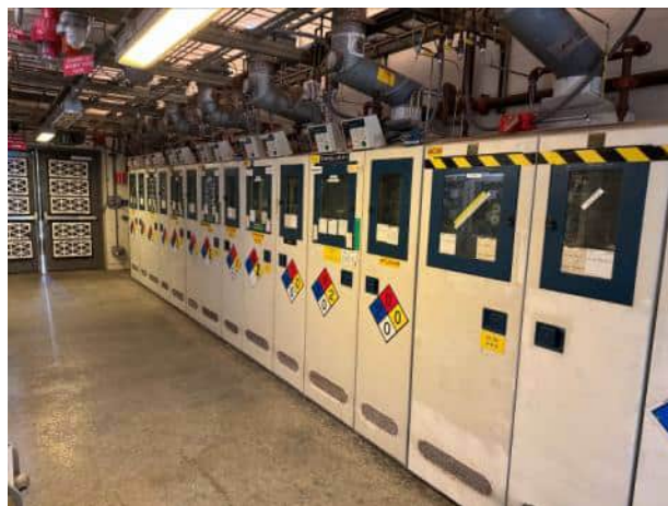
24. View of compressed gas storage
