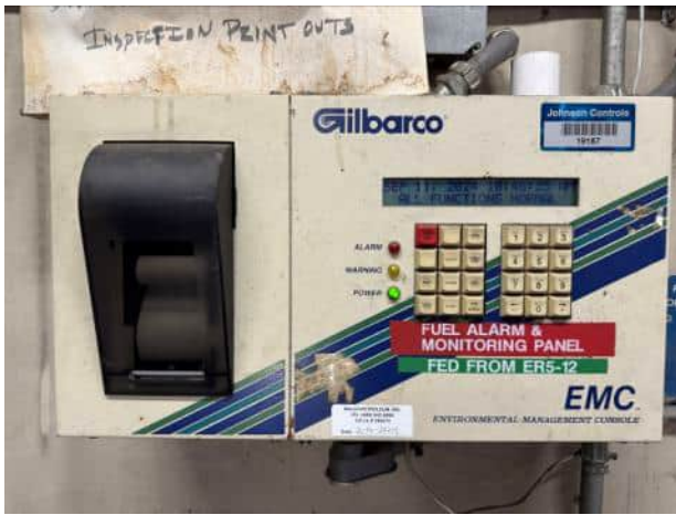
31. View of the UST monitoring system
