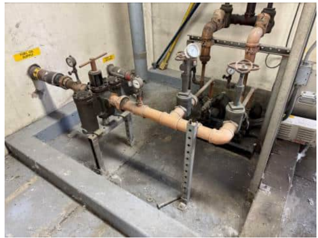
32. View of diesel transfer pumps for the UST and ASTs
