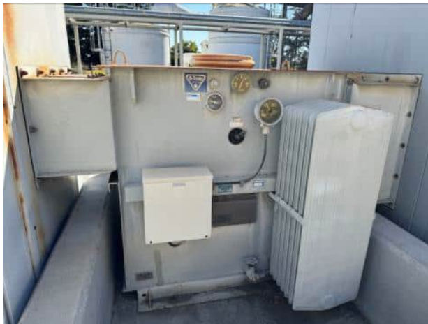
25. View of a transformer
