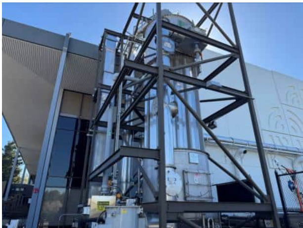
17. View of the arsenic scrubber
