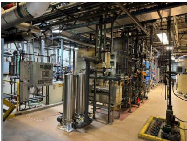
11. View of the water and wastewater treatment systems
