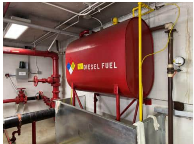
34. View of the fire pump AST
