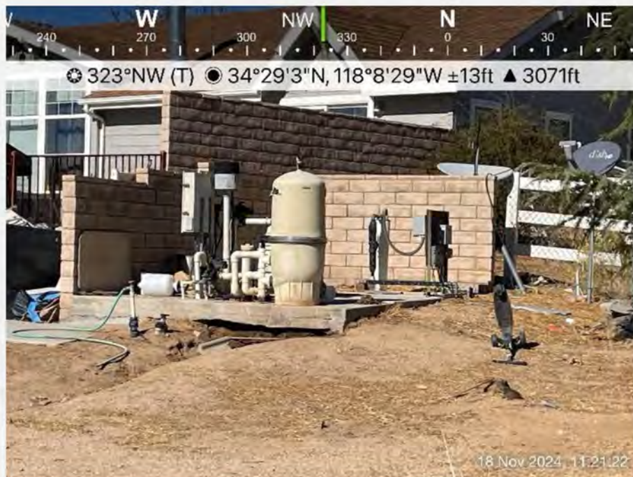
30. Groundwater well located on APN 3056-019-026; provides potable water to the residence located on the parcel.
