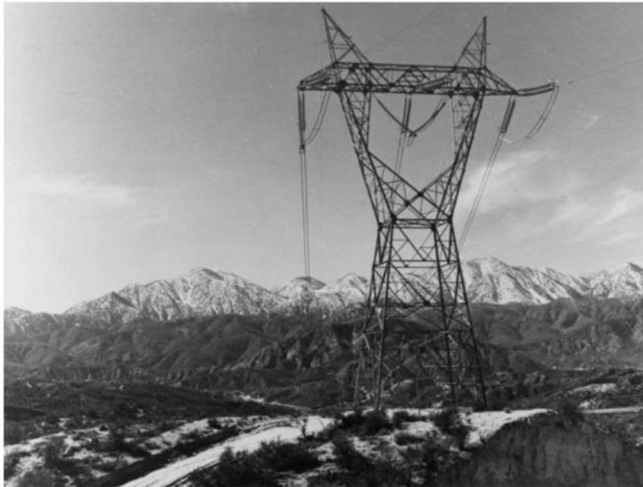
Exhibit 1. Typical SCE 500kV transmission tower, circa 1973
