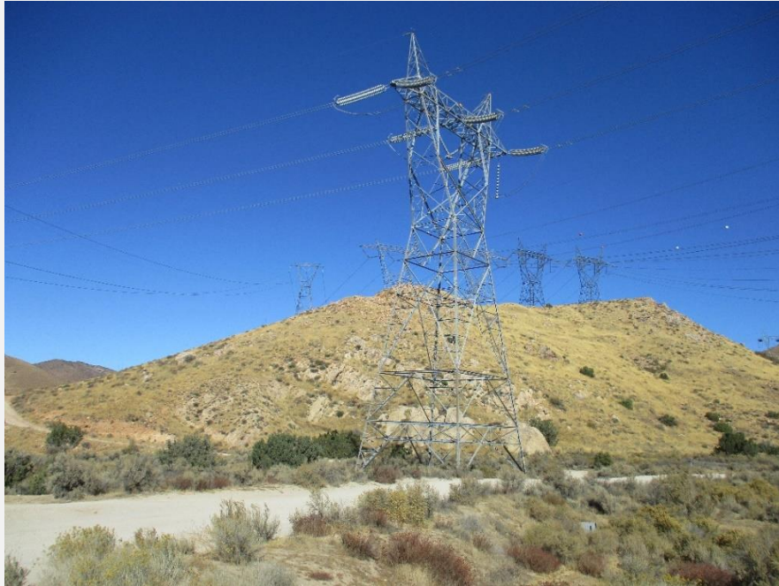
Photograph 3. Representative 500kV tower; Vincent-Lugo No. 1 and No. 2 towers are visible in the background, view looking northeast 12/8/2024
