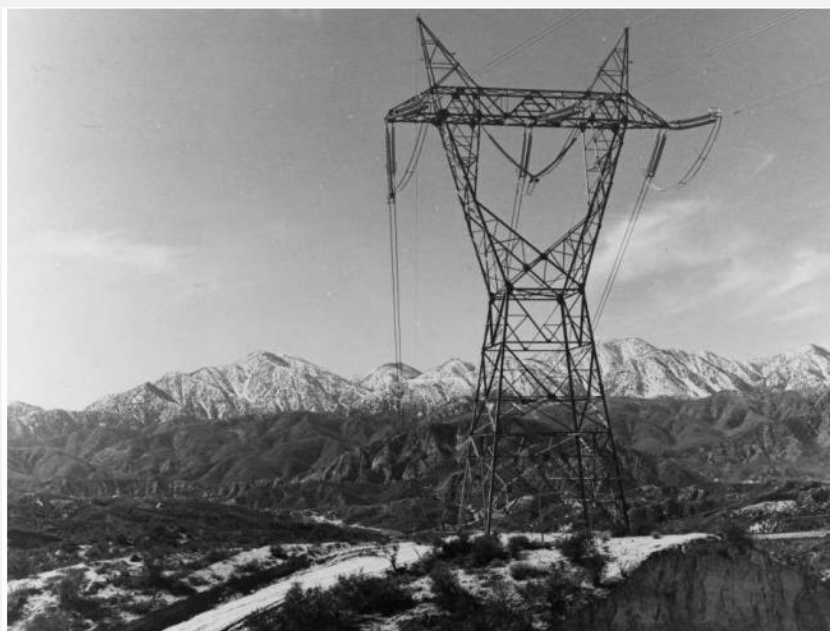
Exhibit 4. Typical SCE 500kV transmission tower, circa 1973.
