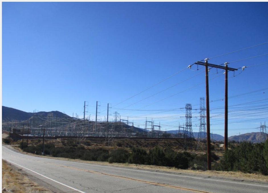
Photograph 2. SCE Vincent Substation, view to the southwest
