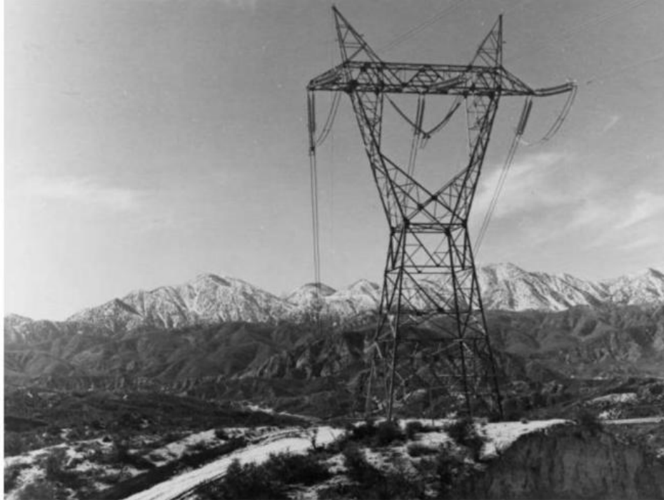
Exhibit 2. Typical SCE 500kV transmission tower, circa 1973
