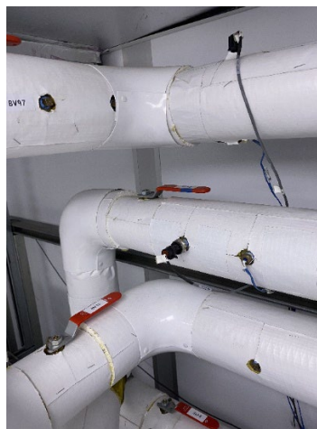
Figure 5-7: Continuous Pipe Insulation
