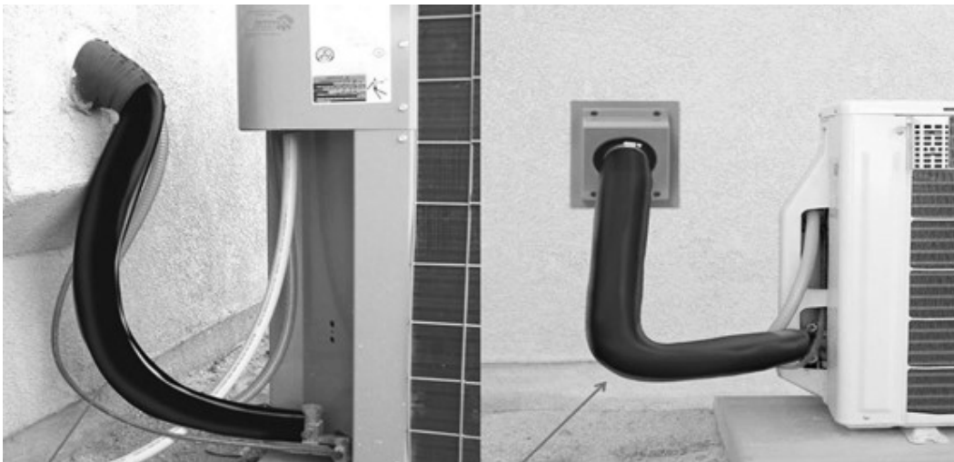
Figure 4-16: Refrigerant Line Insulation
